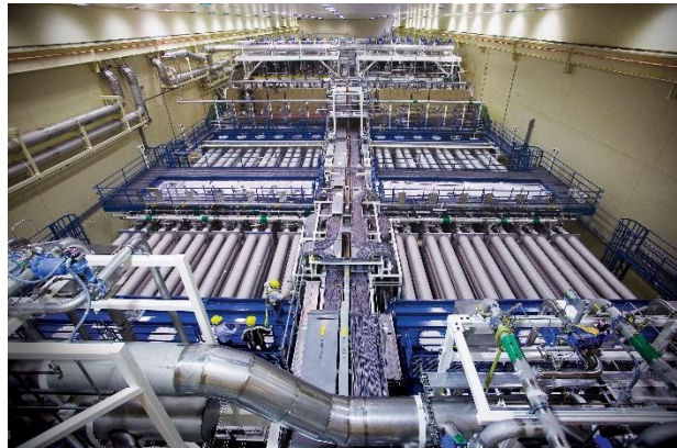
Figure 12. Photo of 1.8MJ laser bay of the National Ignition Facility at Lawrence Livermore National Laboratory.
